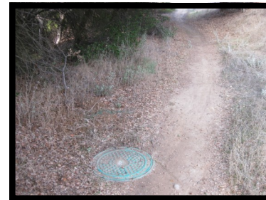
19. Manhole #307 On left side of the path, flush with the ground, North of Balboa Ave.
