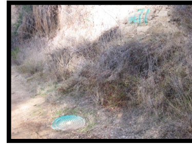
15. Manhole #71 On path to right, flush with ground, North of Balboa Ave.
